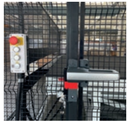
Doors interlocked with a safety lock.
